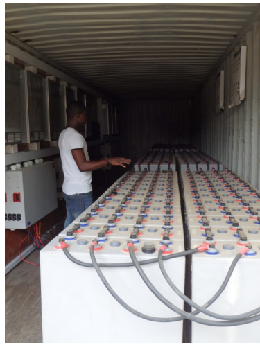
Abdule Mansaray, Panguma's new electrician for solar.
